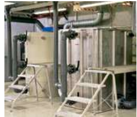
Level measurement in a water treatment plant
